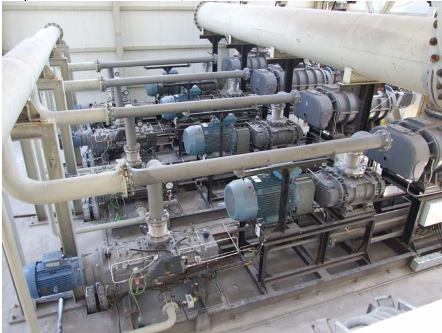
Fig. 4. Typical modular dry mechanical vacuum installation for 90 tonnes VD
